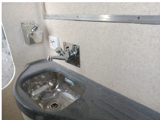
Installed with jaguar fittings
