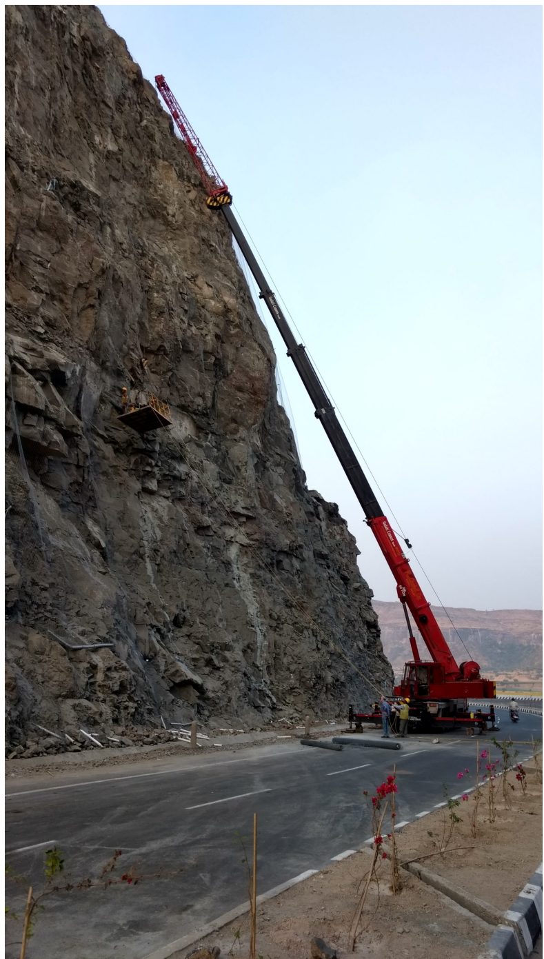
Rockfall protection system
