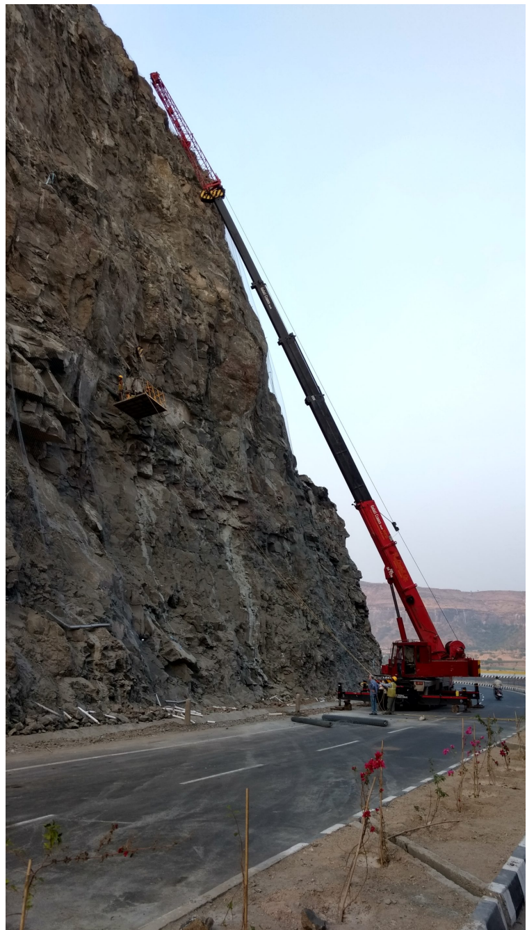
Rockfall protection system
