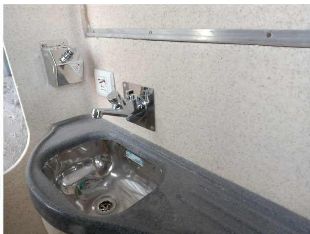
Installed with jaguar fittings
